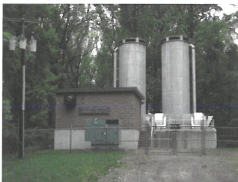
Above: Water aeration plant near Trotter Tract
